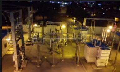
(b) Image Pipes.I, MOS: 2.500
